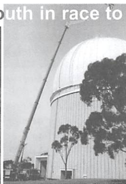
nears the end of the installation phase, ready for first light alongside its older cousin (see also next page).
